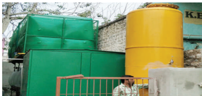
Biogas plant at Kurnool Vegetable Market Yard, Kurnool for the treatment of 500 kg/day of market and vegetable waste
