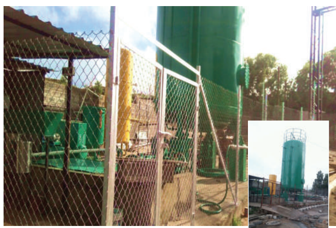
Fig. 17: Full scale biogas plant for the treatment of food waste based on AGR at Hubli, Ahmadabad, Surat and Bhavnagar
