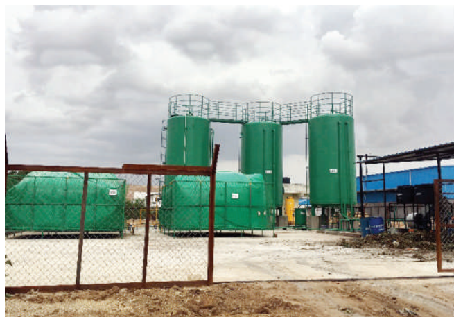
Biogas plant for the treatment of 3,000 – 5,000 kg/day of organic fraction of MSW, installed at Jawahar Nagar, MSW Processing Site, Hyderabad
