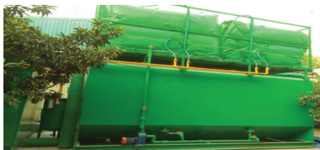
Biogas plant at CapGemini, Hyderabad for the treatment of 250 kg/day of food waste
