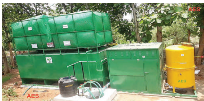
Biogas plant at Odisha for the treatment of 250 kg/day of food waste
