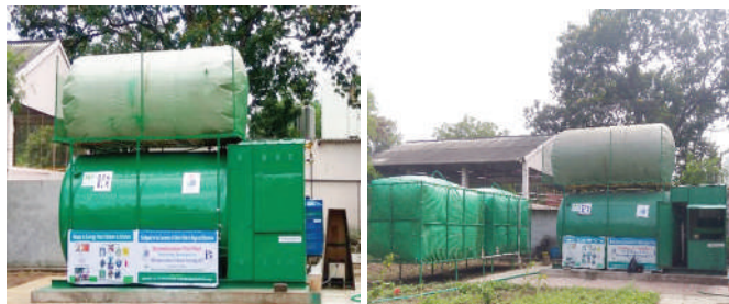
Biogas plant (250 kg/day) installed at CSIR-IICT, Hyderabad
