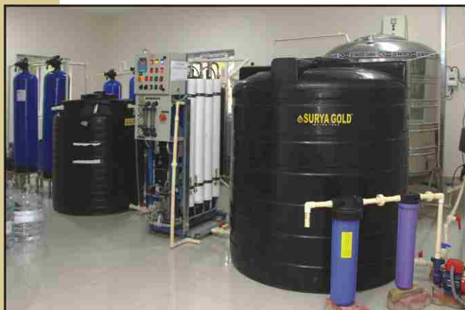
Water purification system
